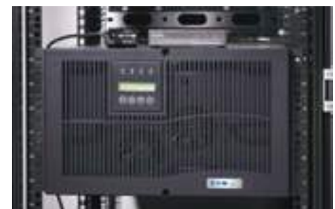
Environmental Monitoring Probe and Environmental Rack Monitor mounted on top of Eaton UPS
