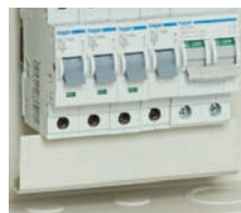
Outgoing devices • Single pole MCB's • 2 module RCCB (split load) • Single pole RCBO
