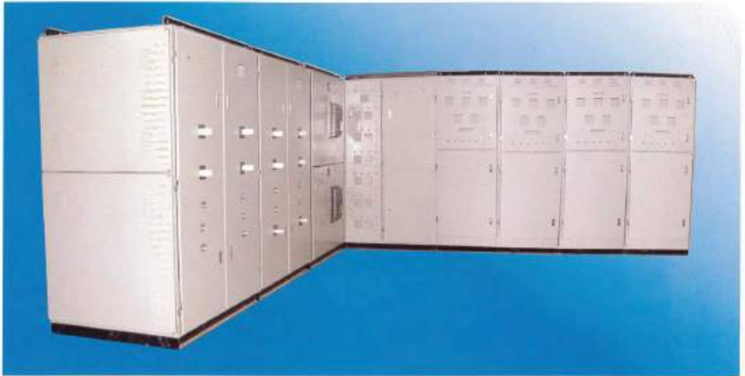
并車櫃 Panels for power supply from several generators join together
