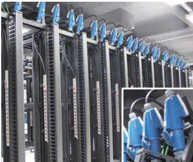
Internet Data Center – South Korea
