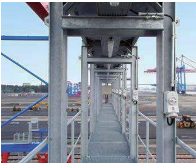
Container Terminal, Altenwerder – Germany
