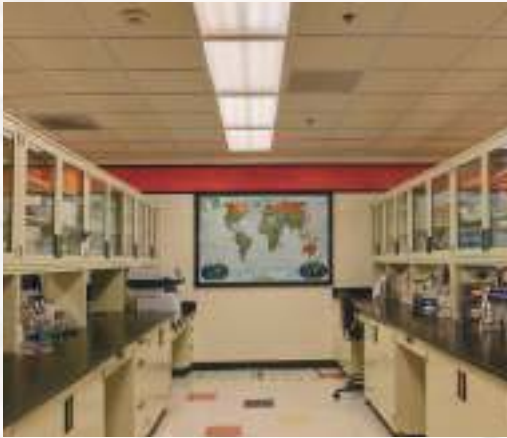
Before: Fluorescent Lighting
