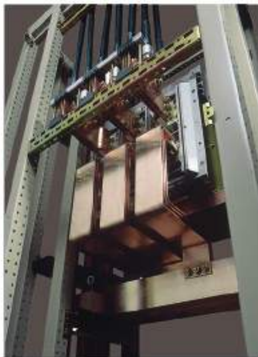
Connection to busbars.
