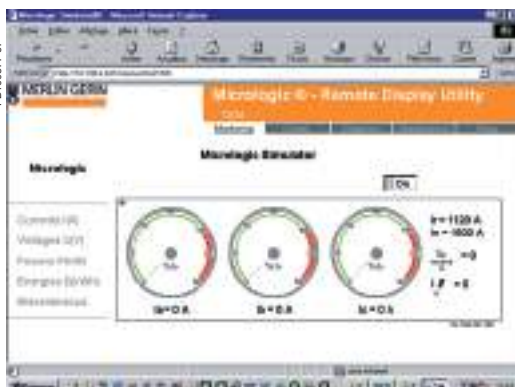
Monitoring of your main LV switchboard via embedded web pages in the MPS100 accessible with a standard web browser.
