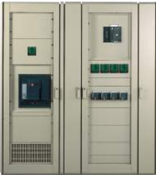
Main LV switchboard.
