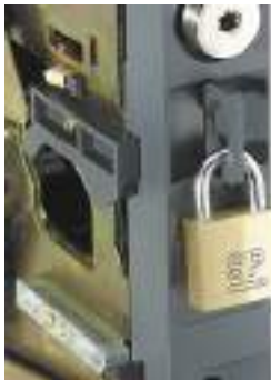
"Disconnected" position locking by padlocks.
